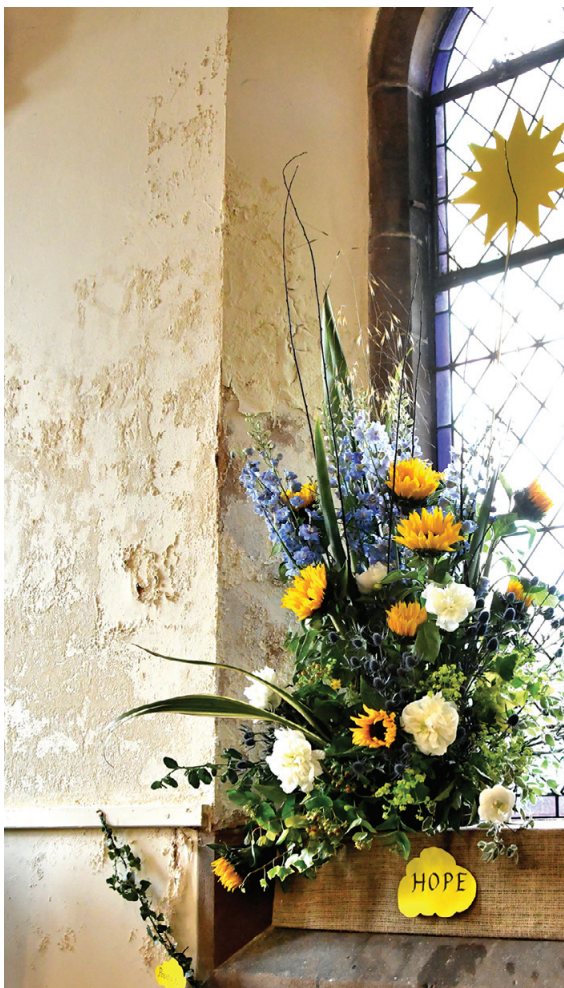
Oulton Church - The photo shows just a small section of major damp issue
