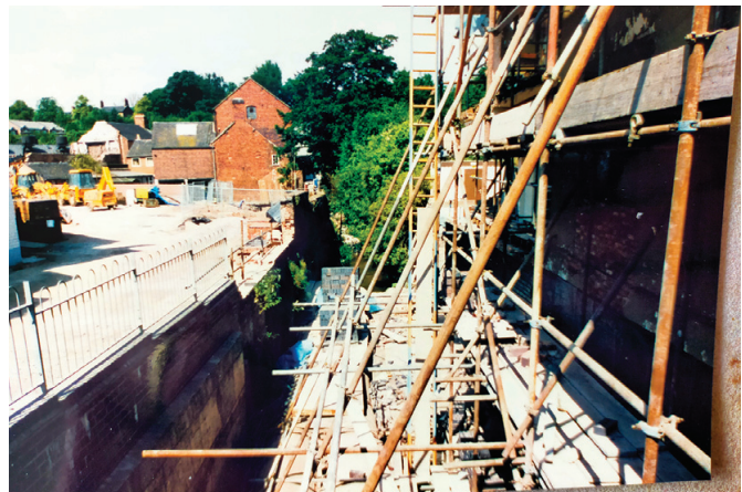
• Strengthening the walls of the building which is now the Post Office
